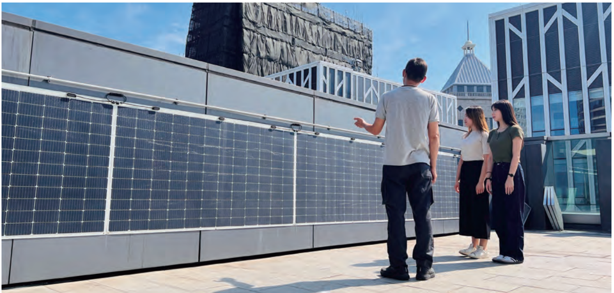
Solar panels were installed at BEA premises to promote renewable energy generation.
